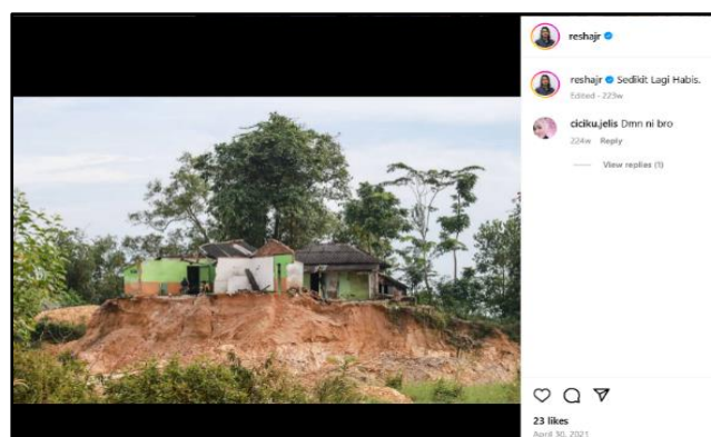
Figure 4. A photograph of several houses that have collapsed or are nearly collapsing due to land subsidence caused by nearby tin mining activities.
